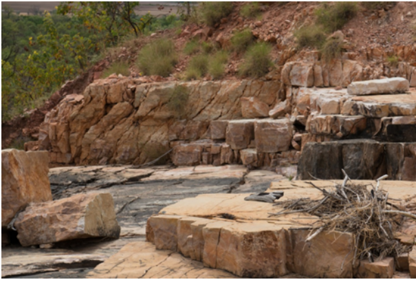
Fig. 3. Moochalabra Dam spillway showing erosion controlled by sub-horizontal bedding and valley stress relief joints in the near surface.
