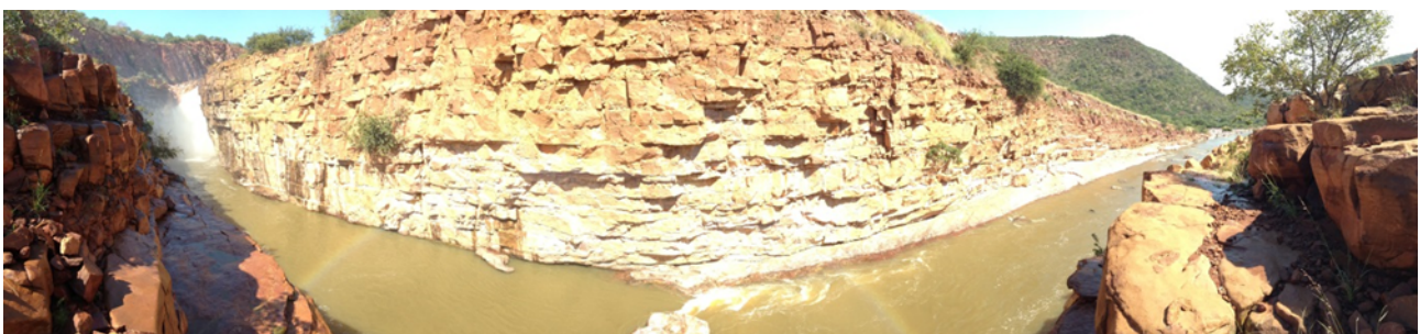
Fig. 8. Mokolo Dam spillway showing erosion up to 25 m deep in fault zone.
