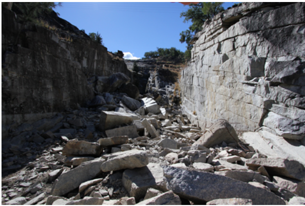
Fig. 7. Copeton Dam spillway showing deep erosion in closely jointed fault zone. Toppling observed in the photo is understood to have occurred post the spilling event. Sheet joints are shown in the walls.
