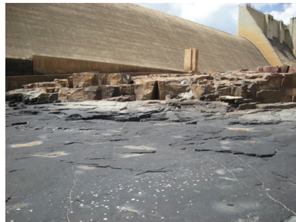
Fig. 11. Burdekin Falls spillway showing remnant jointed rock, and persistent sub-horizontal defects in ignimbrite. The non-eroded area is characterized by having widely spaced tight joints with no free faces to form kinematically viable blocks.
