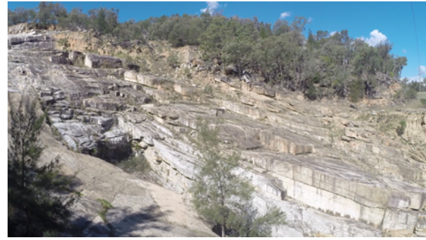
Fig. 5. Copeton Dam spillway showing sheet jointing in granite sub-parallel to ground surface controlling erosion.
