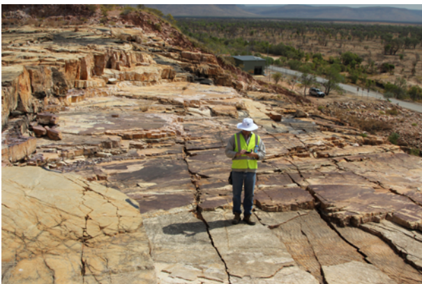
Fig. 4. Moochalabra Dam spillway showing head cutting in sub-horizontally bedded sedimentary rocks exhibiting head cutting at the downstream faces, but resistance to erosion elsewhere.
