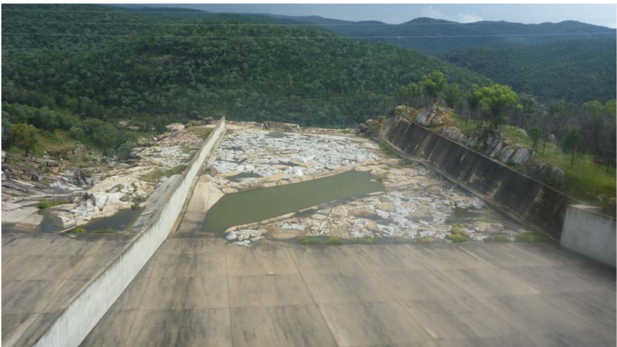
Figure 46 – A the void (see ponded region) formed after a wedge of rock was removed in the service spillway at Copeton Dam (NSW) was lined with concrete, which has proven effective
