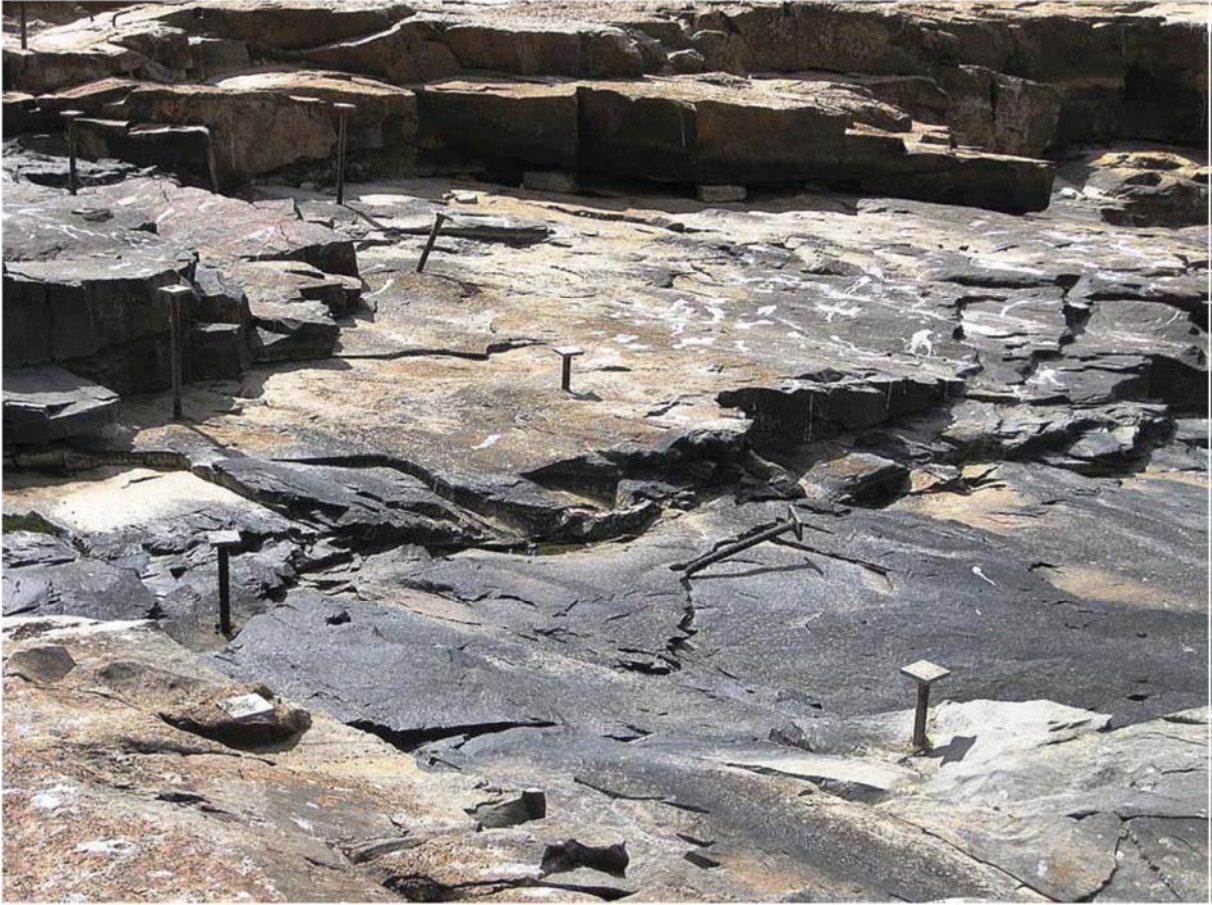
Figure 49 – The spacing for pattern bolting at Burdekin Falls Dam (Australia) exceeded the fracture frequency of ‘capping’ material, and was ineffective in stopping removal of individual rocks (photo courtesy of Sunwater)
