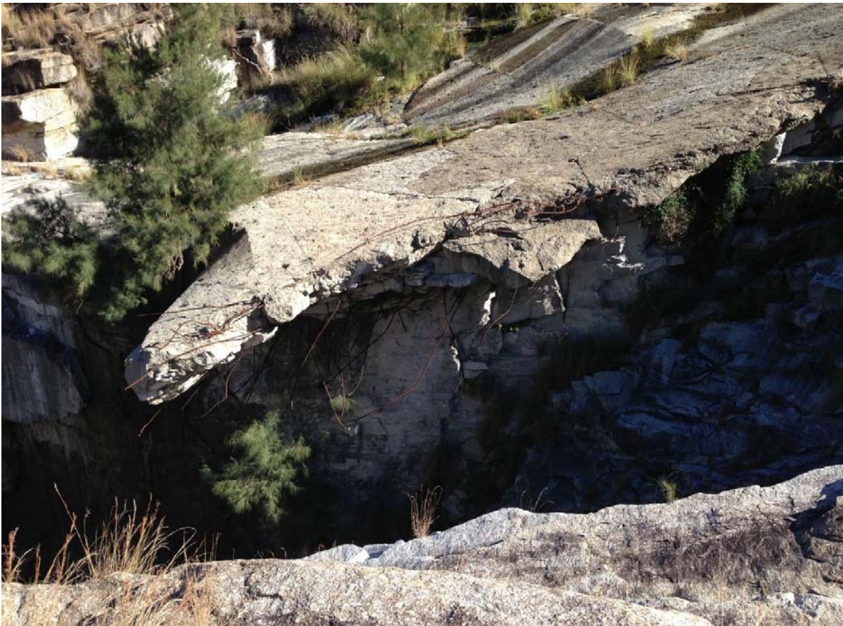
Figure 48 – Concrete lining placed within the erosion gully of the secondary spillway at Copeton Dam (Australia) was of insufficient extent to stop further headcutting occurring during test flows (photo SE Pells)
