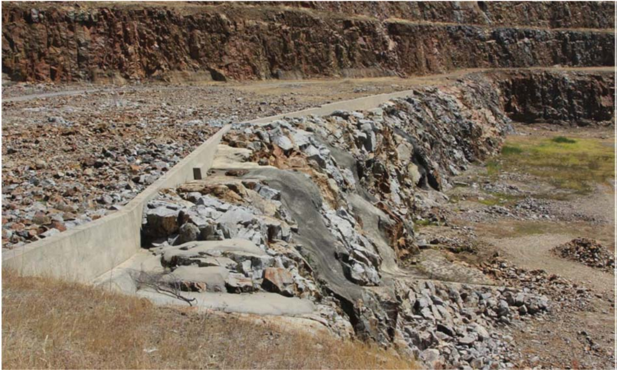
Figure 45 – Placement of concrete sills to distribute flows over unlined cascades at Dartmouth Dam, preventing further channelisation
