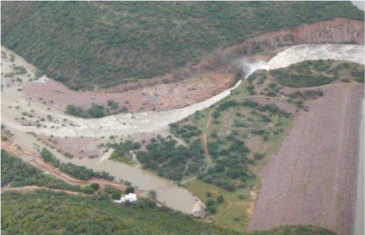
Figure 43 – Stream power dissipation was concentrated into a developed erosion channel at Mokolo Dam (South Africa, photo courtest of M. van Schalkwky).
