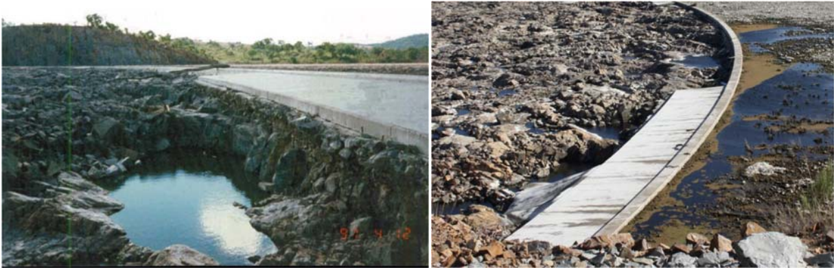
Figure 47 – Placement of dental concrete to fill a void left by erosion of blast-damaged rock at Pindari Dam (Australia) has proven effective
