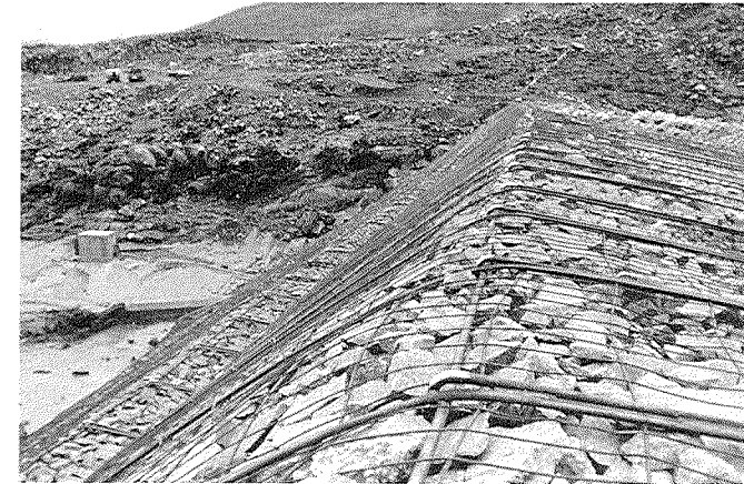
FIG. 8.—Reinforced Rockfill Prior to Flood
